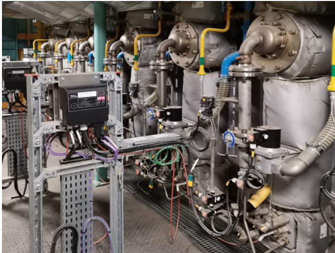
UNI-RAD system with plug-in-recuperator in a W-shaped radiant tube on a strip galvanising line
