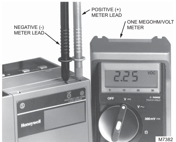
Fig. 5. Measuring 7800 SERIES Control flame signal voltage.
