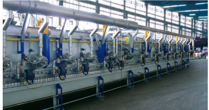
Tailored blank furnace
