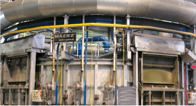
Rotary table furnace
