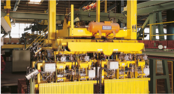
Stainless steel bellows units at the kiln in a brickworks
