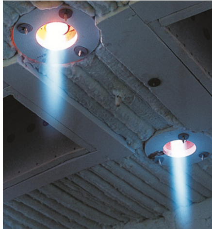
Overhead heating with burner BIC
