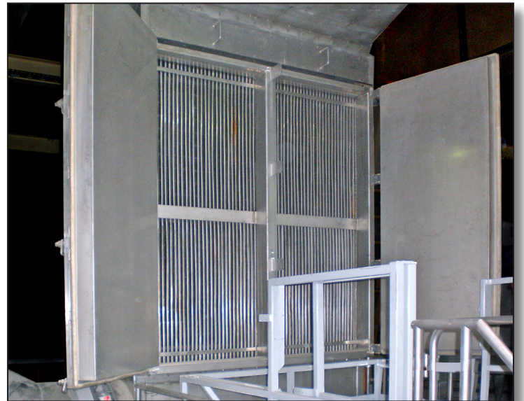
Heat Exchanger With Open Inspection Doors
