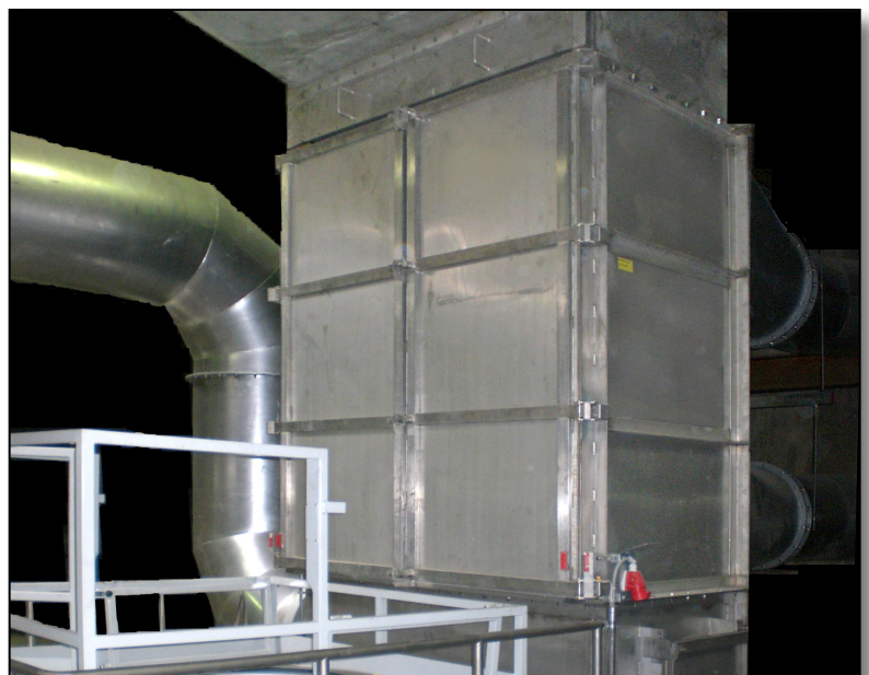
Front Side of Heat Exchanger With Inspection Doors Closed
