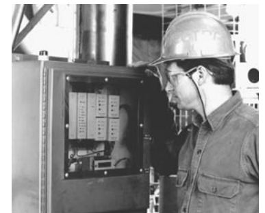
Vectra Fitness engineer checks Multi-Flame monitoring system that's performed flawlessly since its installation two years ago.
