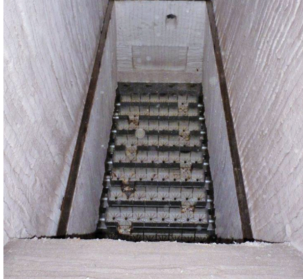
Interior view of the heating duct showing the Eclipse RatioStar burner configuration.
