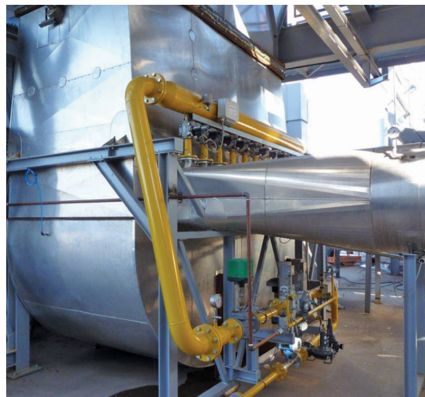
Exterior view of the heating duct showing the Eclipse gas train that supplies the RatioStar burners.
