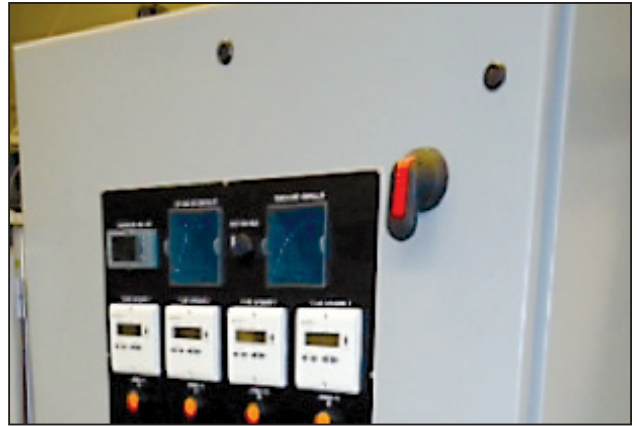
Burner management panels.
