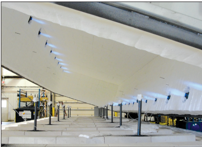
During the initial test firing with the furnace operating at 2000°F, the exhaust temperature test readings were 430°F, exactly as predicted by Eclipse.
