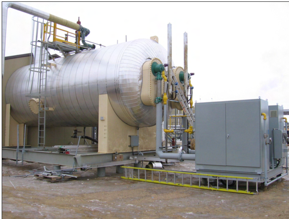
Overall Side View of Unit Showing Both IJ-8 Burners and Control Cabinets
