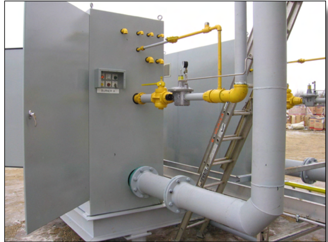
Cabinet End View
