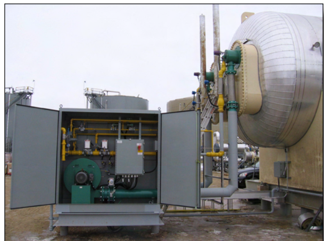
Combustion Cabinet Inside
