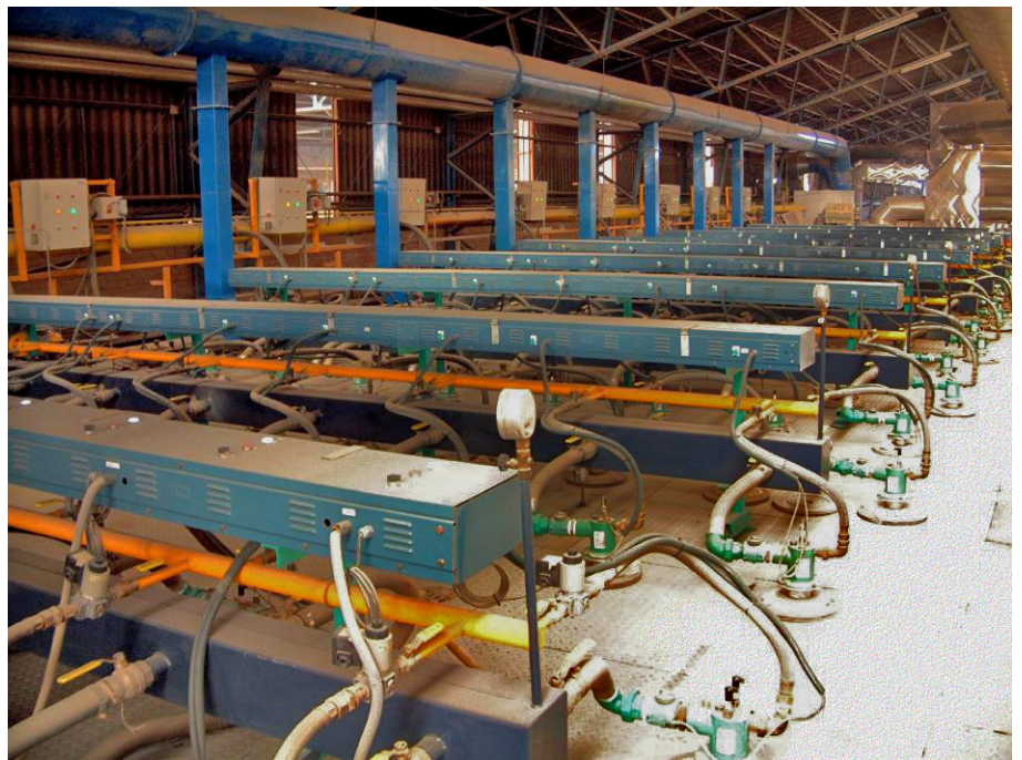
Additional view showing combustion air supply lines and electrical wiring.
