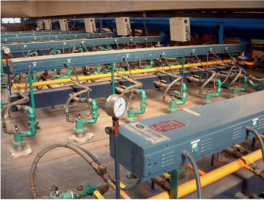
Roof mounted Eclipse ExtensoJet burners on the heating zone of the furnace.
