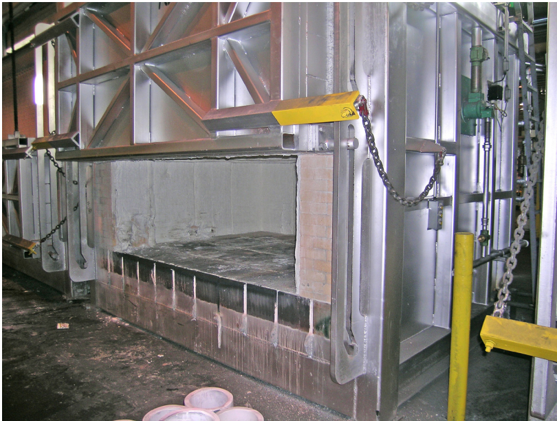
New forging furnace showing one of two Eclipse Furnnox burners.
