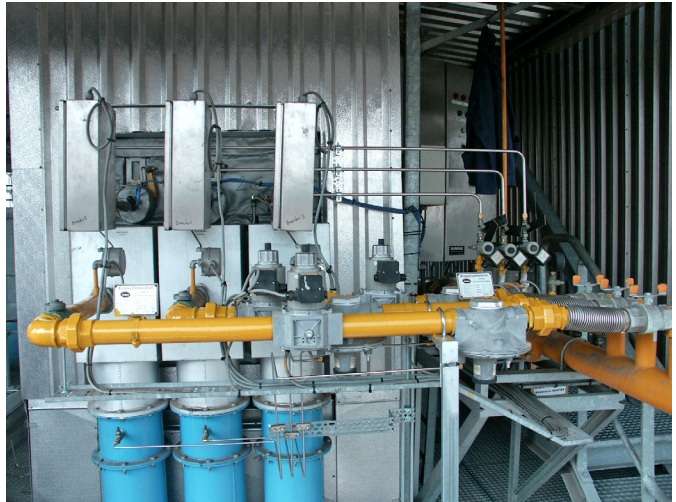
Burners with UV cells, gas train and combustion air duct
