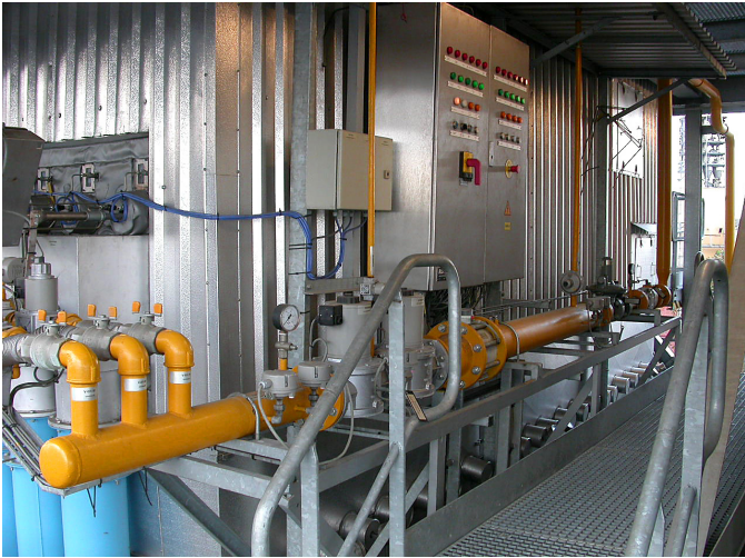
Gas train and control panel
