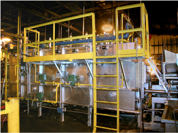
Side view after upgrade showing gas piping
