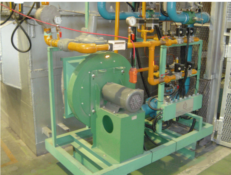
Close Up of Gas Train
