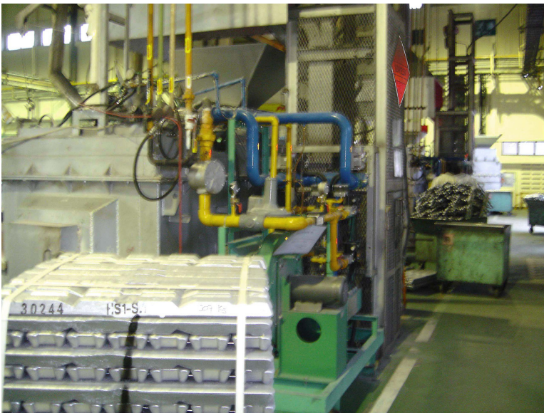
Gas Train System
