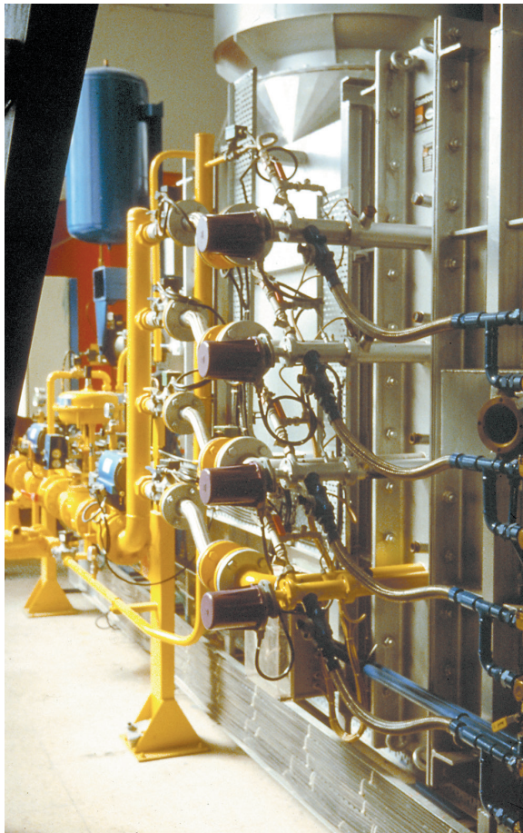
FlueFire system installed in a cogeneration plant
