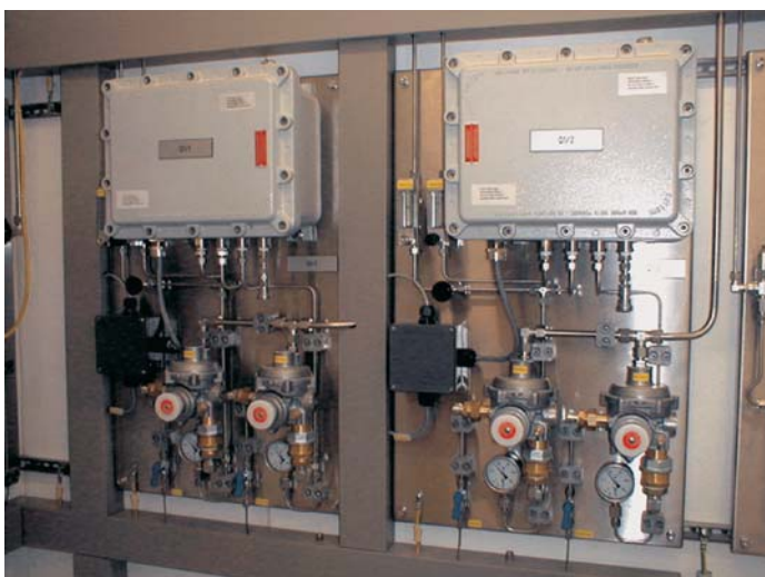
Bild 7: 1v2 Gasbeschaffenheitsmessung in Gasmischstation Weine Fig. 7: One-from-two gas-quality measurement at the Weine gas mixing station
