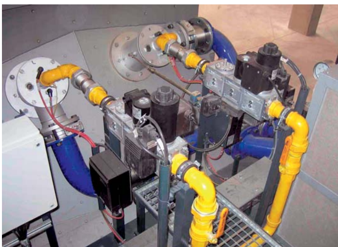
Fig. 1: Typical layout of a heating system with pneumatic air/gas ratio control system
