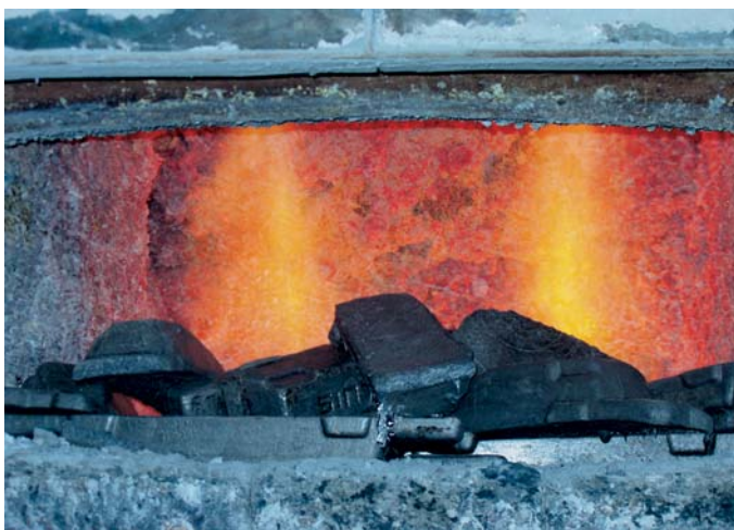
Fig. 3: Aluminium smelting furnace at high-fire rate. The furnace is charged with aluminium ingots. It is fired by two Elster Krom-schröder burners ZIO 165 with a rated output per burner of 630 kW
