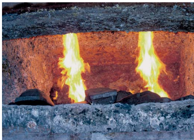
Fig. 4: Aluminium smelting furnace at low-fire rate. The furnace is charged with aluminium ingots. It is fired by two Elster Krom-schröder burners ZIO 165 with a rated output per burner of 630 kW
