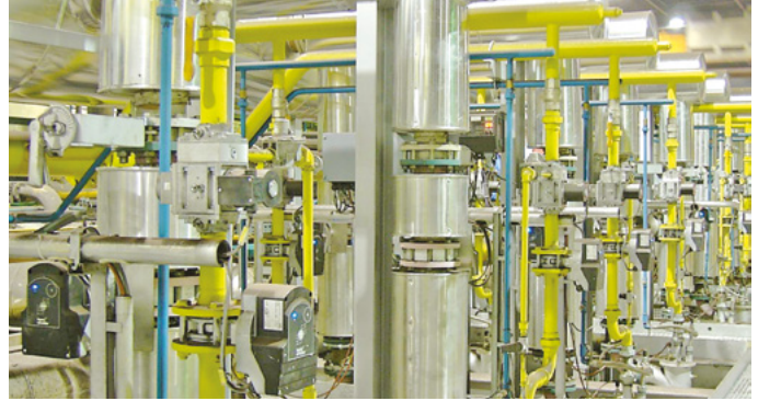
Walking beam furnace with overhead firing
