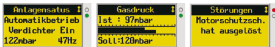
Fig. 7: Status display of the control system
